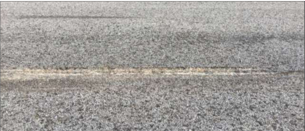
Runway surface scraped by LH wheel after tyre burst
