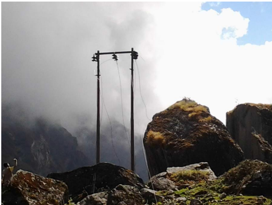
CABLE (WHICH WAS HIT BY HELICOPTER) RUNNING ACROSS THE ABANDONED POLE
