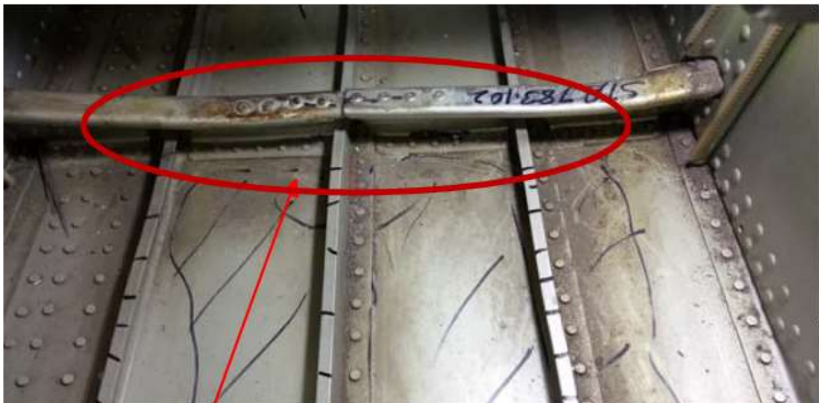
Buckling damage at Frame X783.602
