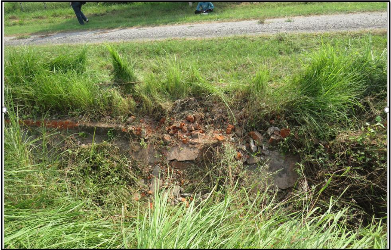
Fig: Damaged Monsoon Drain
