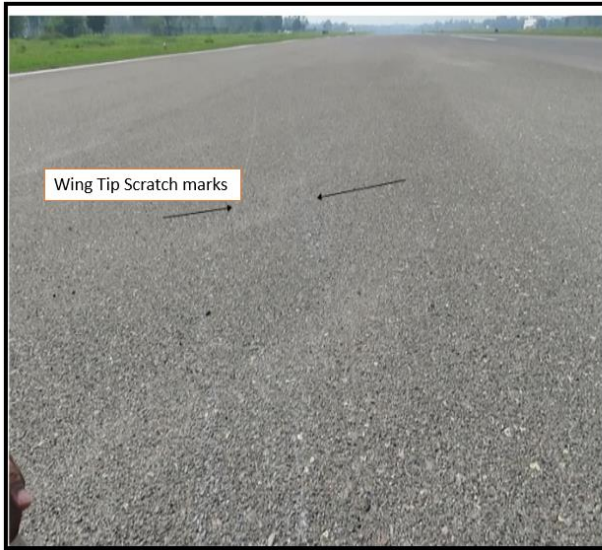
Wing Tip Scratch Marks on Runway
