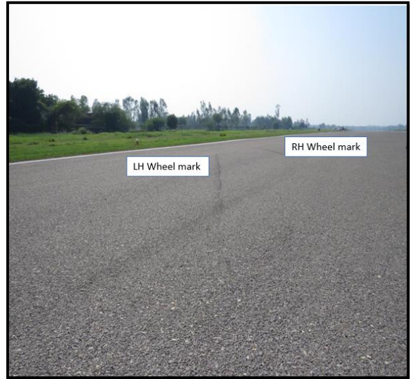
MLG Tyre marks on Runway
