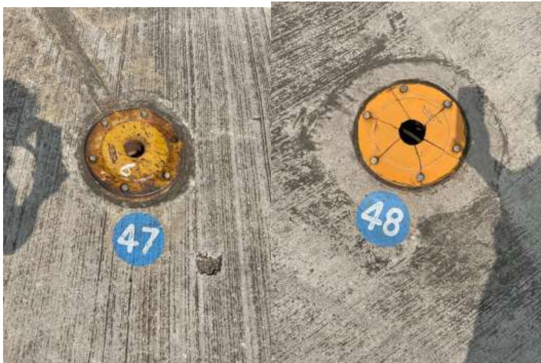
Figure: Missing Edge lights in point of accident
