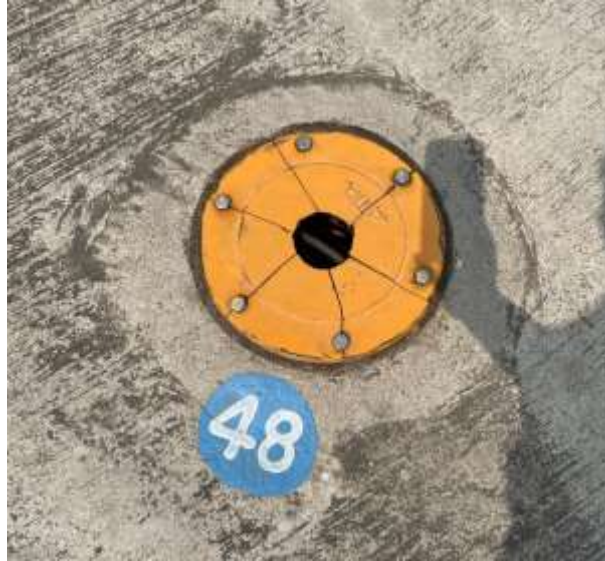
FIGURE: MISSING TAXIWAY SHOULDER LIGHTS (at the time of accident)
