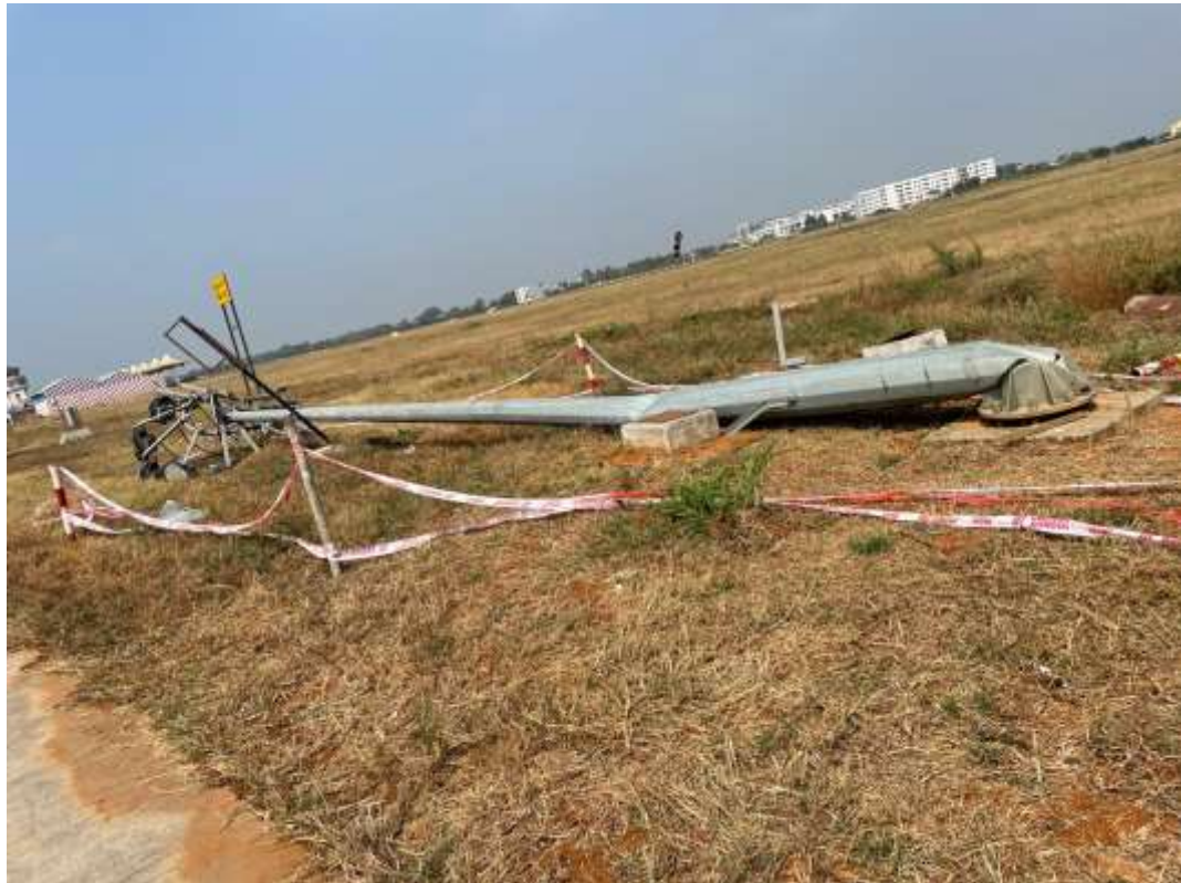
Figure: Damaged Flood Light Mast
