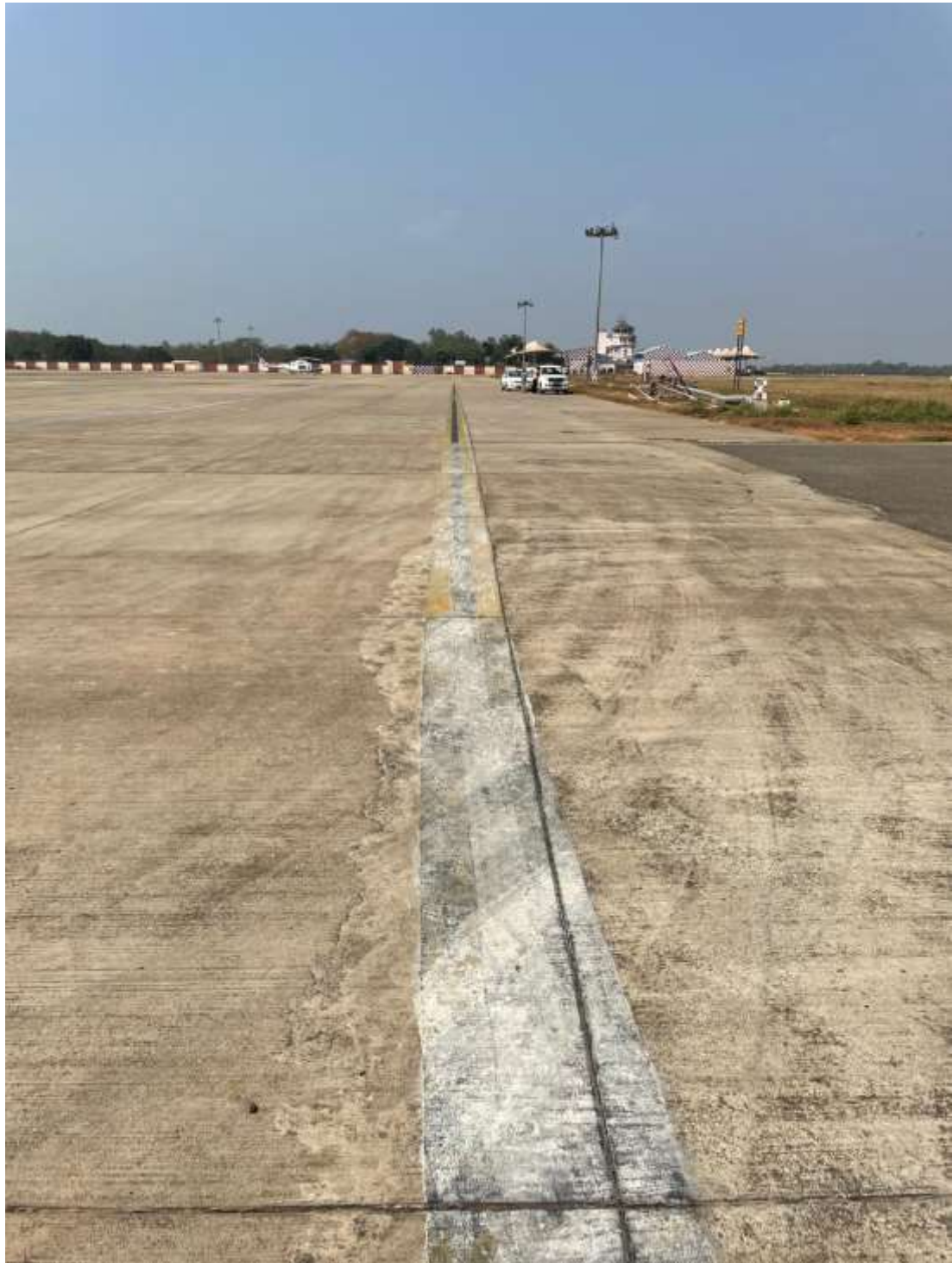
Figure: Existing marking of erased portion at Vijayawada Airport
