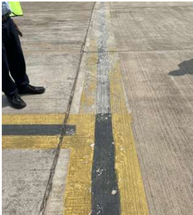
FIGURE : INAPPROPRIATE MARKING AT SHOULDER
