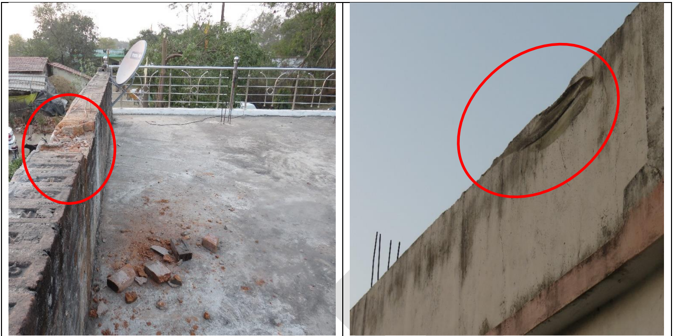
Fig 3 & 4: Third Impact with concrete terrace of a building and landing gear impact marks
