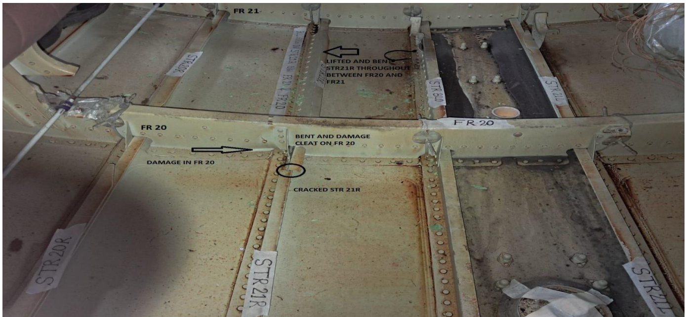
Figure 5. Damage was observed in the lower fuselage structure.
